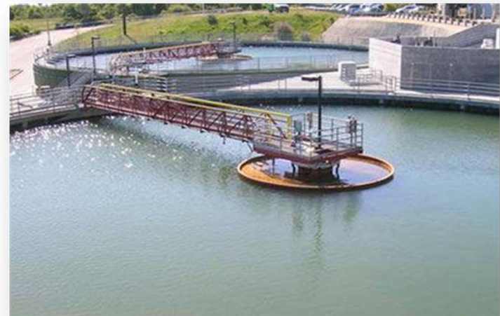
Harry Tracy Water Treatment Plant
