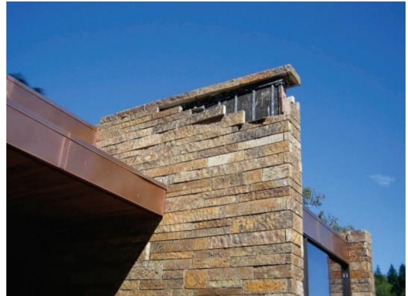
Photo from FEMA E-74
