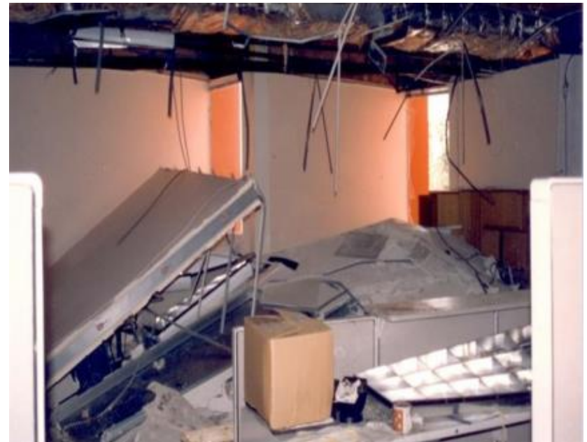
Photo from FEMA E-74
