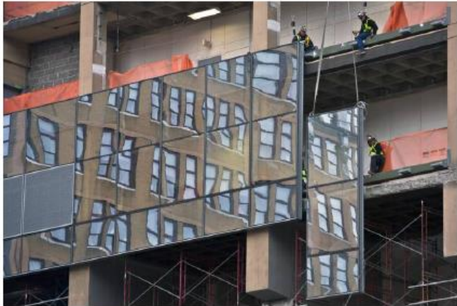
A typical high-rise office tower can need hundreds of thousands of square feet of metal-framed glass panels. A Brookfield Property under construction in New York City. PHOTO: BEBETO MATTHEWS/ASSOCIATED PRESS
