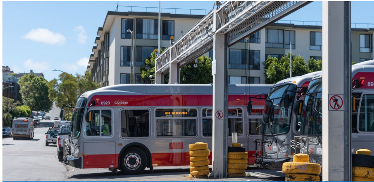
Electrification Infrastructure (Trolley & E-Bus)
