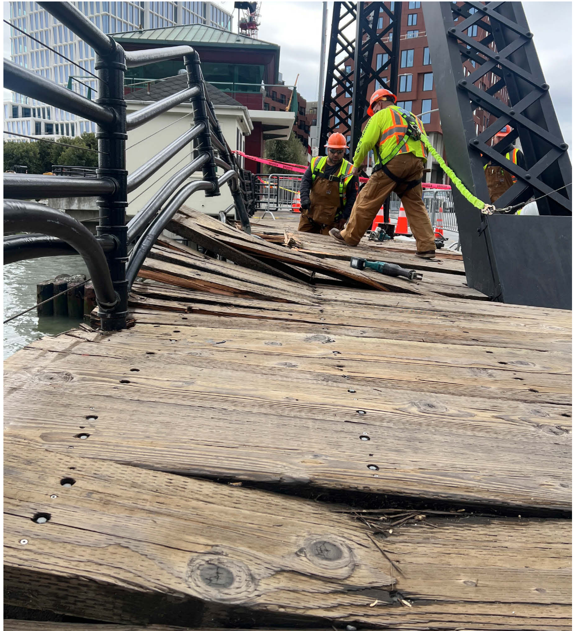
Third Street Bridge Storm Damage
