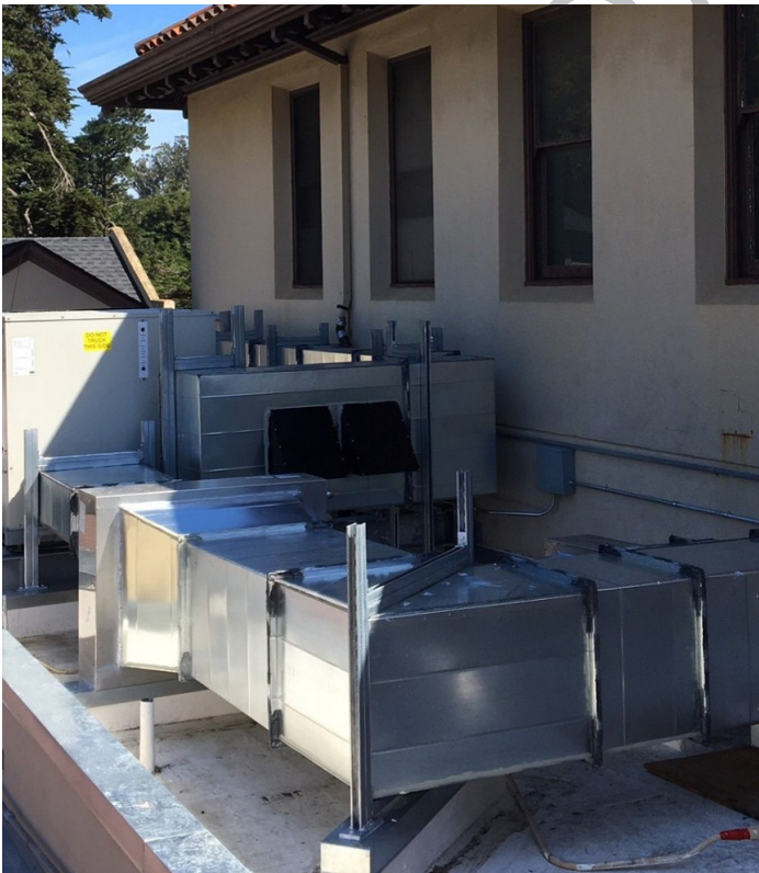
New HVAC unit at Park Station
