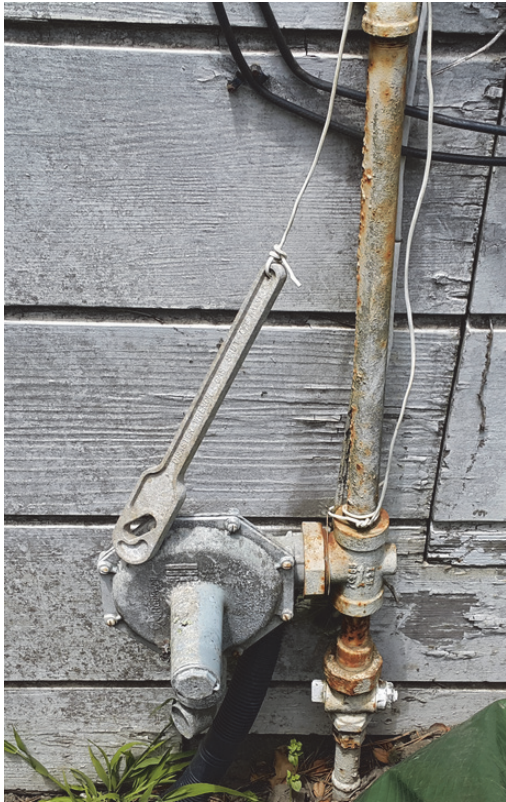
Figure 2-5 “Earthquake wrench” tied to gas line, ready for use.
