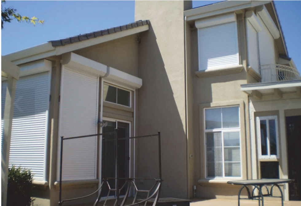
Figure 2-15 Example of protected openings, in this case, roll-down shutters (image from www.ERSshading.com ).
