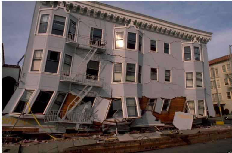
Damage from the 1989 Loma Prieta Earthquake
