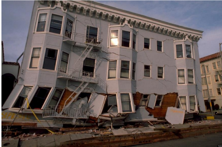
Damage from the 1989 Loma Prieta Earthquake
