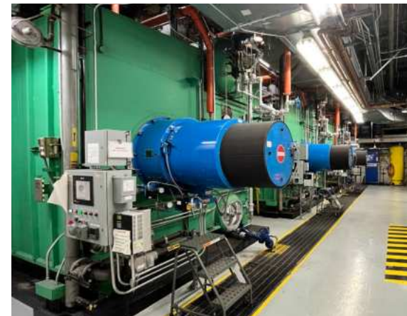
Hall of Justice Boiler
